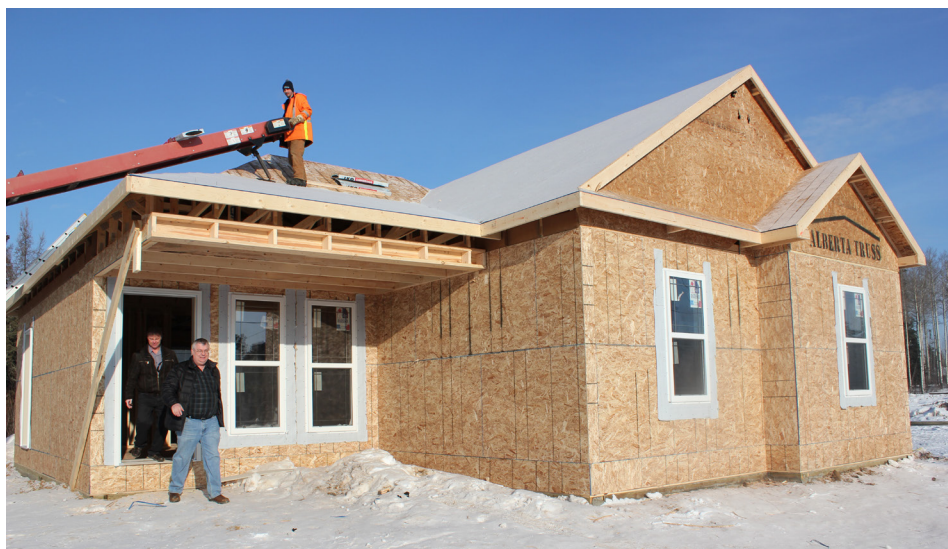
Owen Mitchelmore and Harold Davis inspect one of the many new houses under construction. This one of the dozens of beautiful homes that will be built over the next 3 years in Fort McKay. See Housing Questions Answered on page 2.
