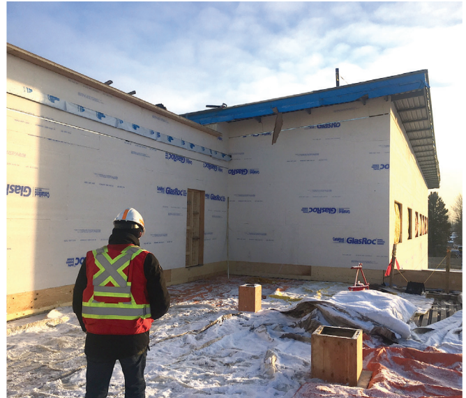
Rick Bouchier, Director of Public Works touring to review work to date on the facility. Rick is maintaining a close connection as major systems are installed and his department is essential for the long-term maintenance of the facility after its completion.
